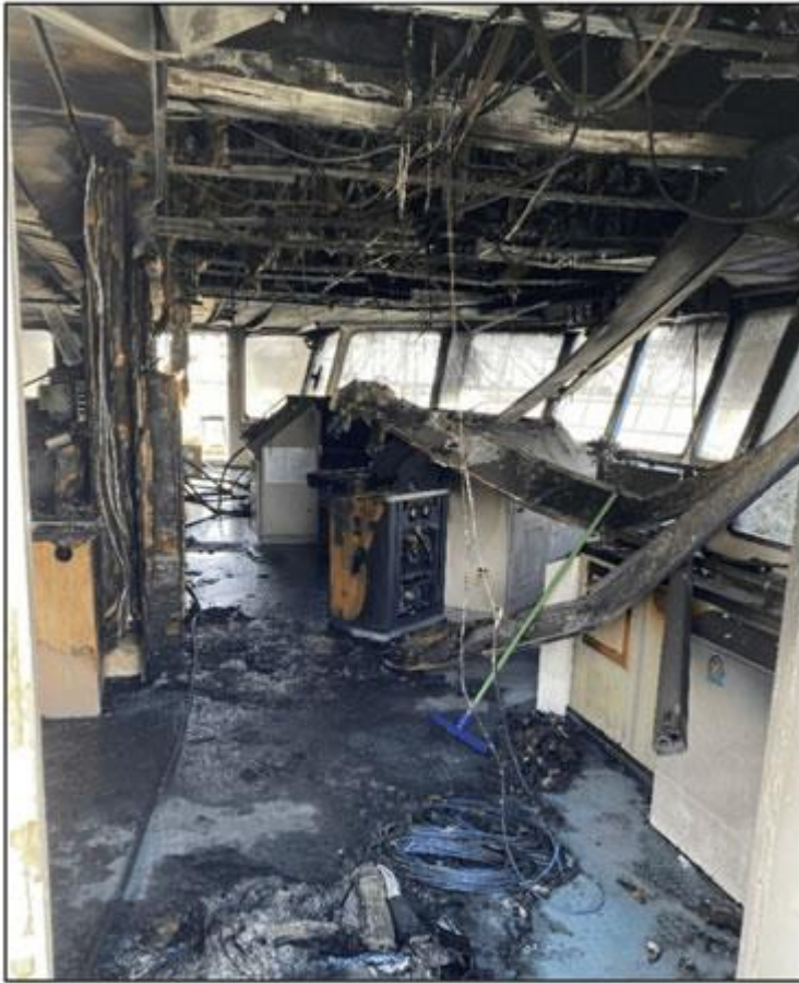
Figure 3. The damage to the bridge. (Source: Coast Guard)
